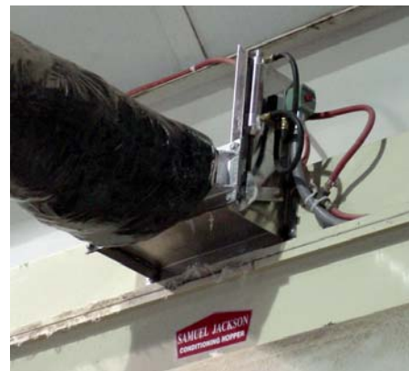
An air-actuated valve stops the flow of moist air to seedcotton when the feeder stops. Note the black Cotton Koozie insulation system being used on the pipe in this system.
