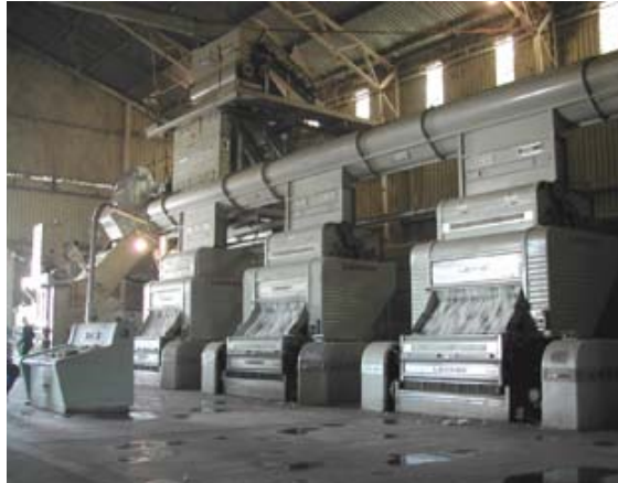
In this photo, moist air is being applied at the feeders. The puddles of water on the floor were from spray to control airborne dust.
