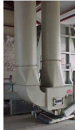
A Hot Box II installed with a fixed head module feeder. Seed cotton travels into the gin with hot air – rocks and green bolls are dropped.
