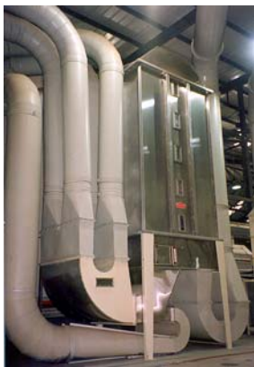
A Fountain Dryer with hot air injection before the inclined cleaner.
