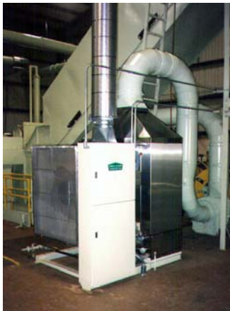
Gas-fired Humidaire Unit
