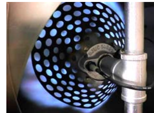
A Samuel Jackson burner provides heated air for the Humidaire's spray chamber
