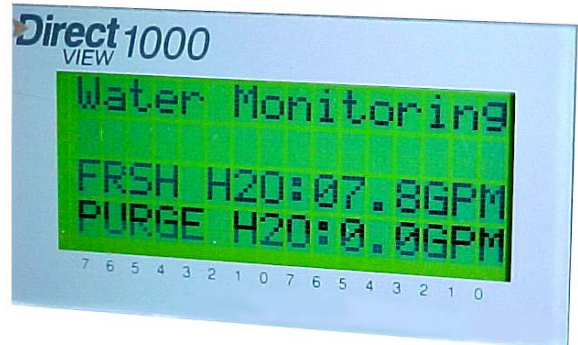
Water usage and flow rates are displayed by the Humidaire Unit's control system.
